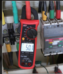
High voltage (600V) frequency measurement
